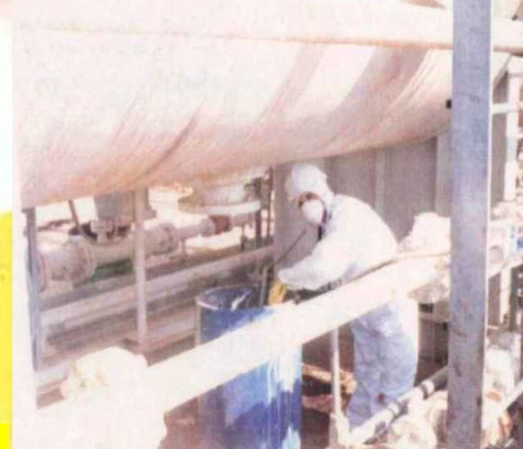
Removal of bulk sludge from a vessel (courtesy: Atomic Energy Commission of Syria).
